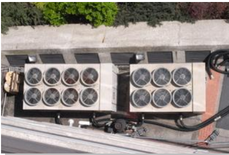
Elevated view of the completed installation
