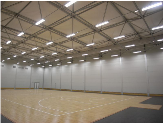
Internal shot of one of the completed basketball courts. One of the 800mm air socks can be seen to the rear
