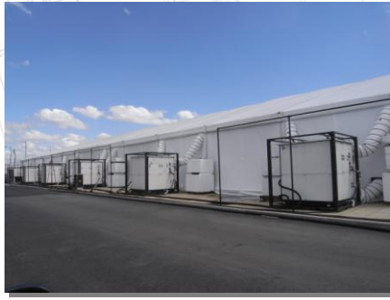
Six ACS 100.60 rental air handlers were fitted.
