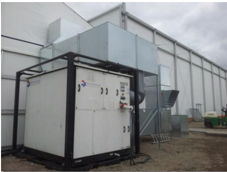
A climate control unit installed with fixed ductwork supplying a light-weight structure (marquee)
