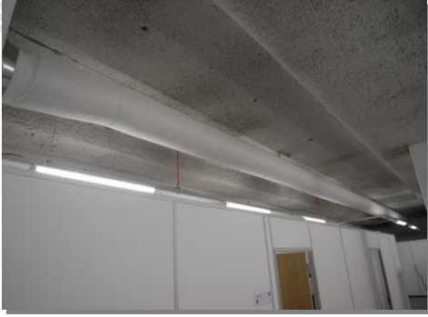
Inside the breakout area. One of the 400mm supply air socks
