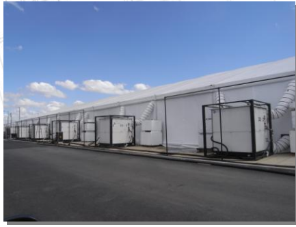
Six ACS 100.60 rental air handlers were fitted.
