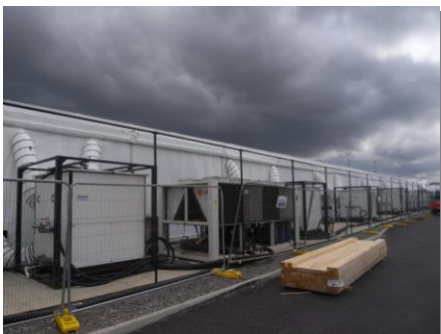
The trane 400kw rental chiller supply the AHU's with cool water
