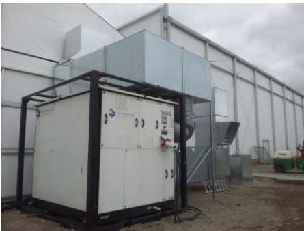
A climate control unit installed with fixed ductwork supplying a light-weight structure (marquee)
